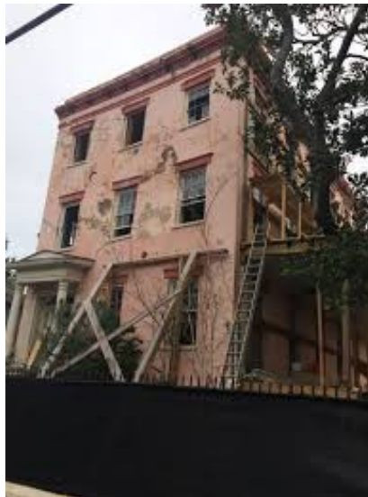
Historic residence stabilized to avoid collapse
